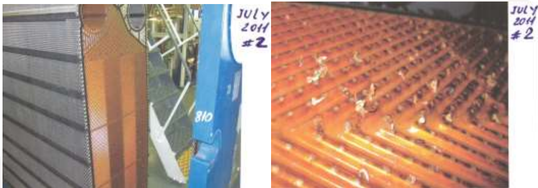
Figure 3. Main Cooling System before – July 2011
