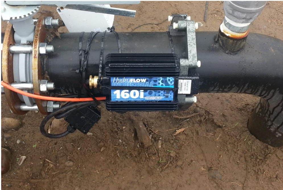
Installed HydroFLOW water conditioner
